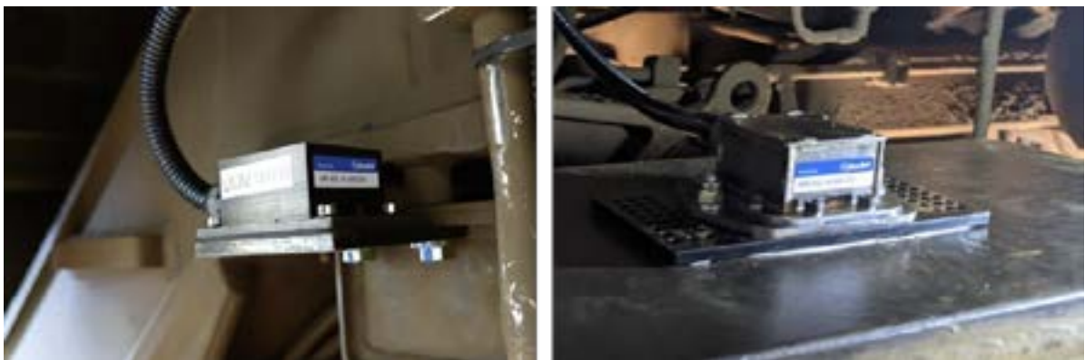
Figure 8: Bogie mounted system on an in-service train (left) using existing fixing points - C374 (right) using adhesive - C170
